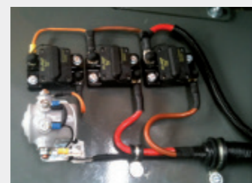
Starter circuit with marine solenoid electrical system with marine circuit breakers replacing main fuses in engine bay
