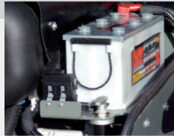
120Amp battery along with battery isolation
